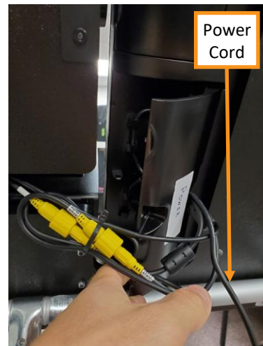
Figure 37. Power Cord connected
